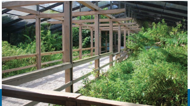
The Living Machine is a green, wastewater treatment facility.
