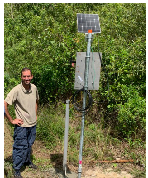
Engineer installing water level recorder.
